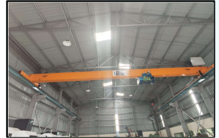
5T Single Girder EOT Crane
