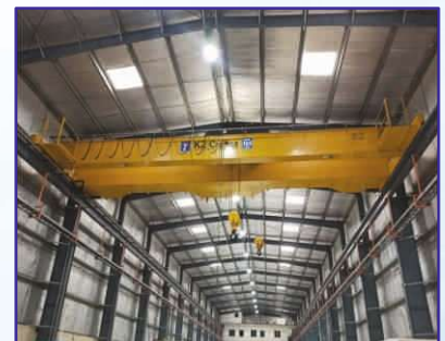
CRANE CAPACITY 16/5Ton & 10Ton CRANE
